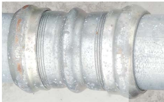
Figure 12 – Example of a threadless coupling (Photo source: Rich Gallagher, Zurich)
