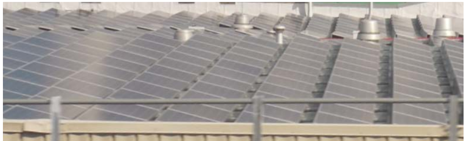
Figure 1 – With the installation of photovoltaic modules, in this example, the presence of rooftop electrics expands considerably compared to the pre-existing rooftop fans (Photo source: Rich Gallagher, Zurich)
