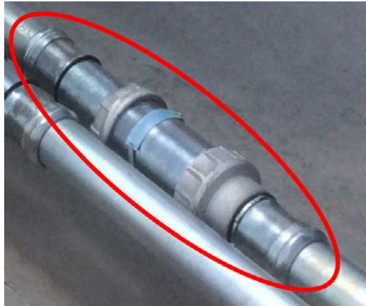
Figure 11 – Example of a conduit expansion coupling (Photo source: Rich Gallagher, Zurich)
