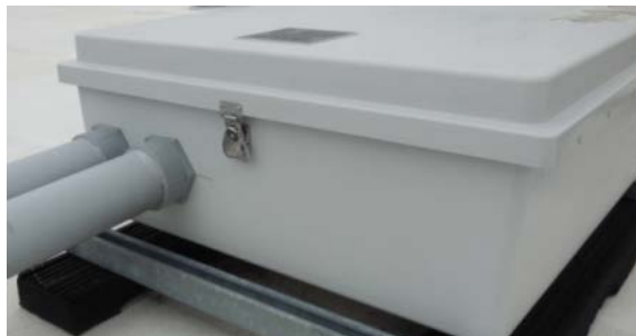
Figure 4 – Junction box (Photo source: Rich Gallagher, Zurich)
