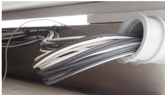
Figure 3 – Insulated cables (Photo source: Rich Gallagher, Zurich)
